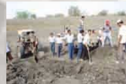
Gabriel Volunteers working actively towards raising ground water levels at Bilawali Talab near Dewas.
